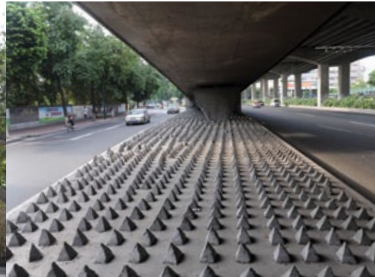
Concrete spikes installed underneath freeway bridges in the city of Guangzhou, apparently intended to deter homeless people from taking up residence. Source: QQ.com/Southern Metropolis Daily
